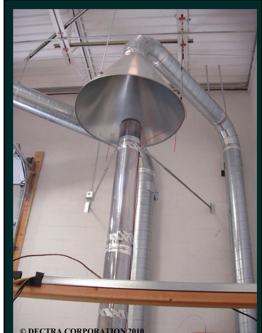
A closer view of the dilution tunnel hood and duct.
