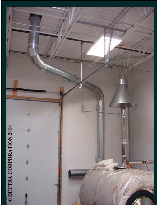
This is an overall view of the hood and duct of the dilution tunnel. The exhaust fan is located on the roof.
